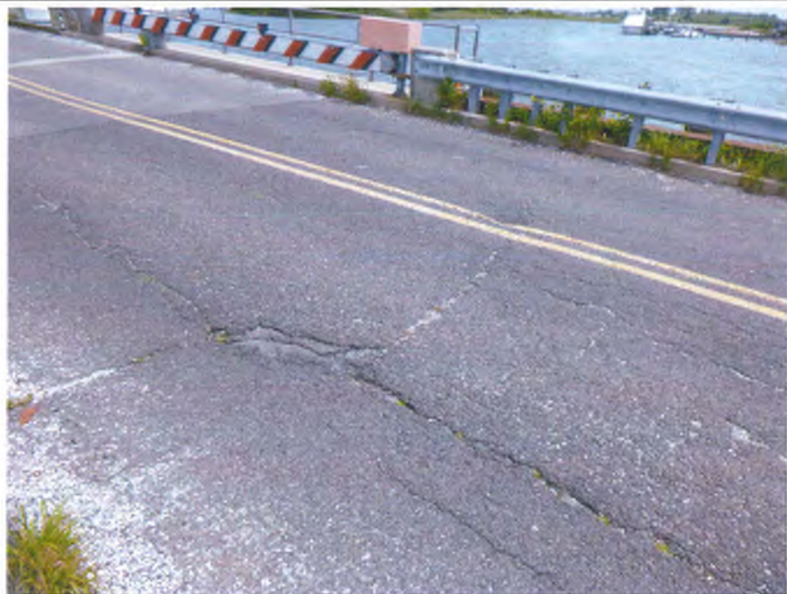
Photo 14 Category: 03 - Roadway, 02 - Approaches Description: West approach roadway, looking southeast. Wide cracks and potholes.
