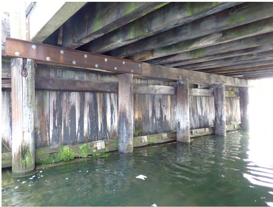
Photo 17 Category: 30 - Abutments Description: North abutment, looking northeast. Deteriorated sheeting. Note the steel channel bolted to the timber pile cap.
