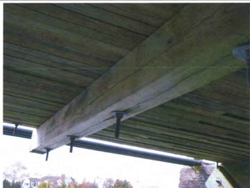
Photo 19 Category: 20 - Superstructure Defects Description: Medium to wide checks in transverse tie in Span 4, looking south.
