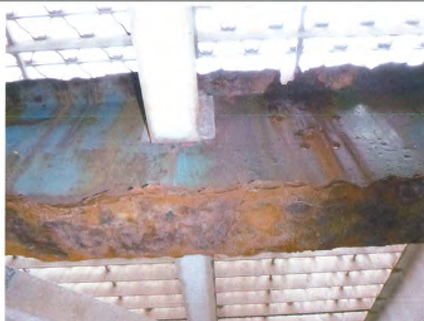
Photo 25 Category: 20 - Superstructure Defects Description: Section loss in top and bottom flange of Floorbeam 2 in Span 6, between Stringers 6 and 7, looking west.
