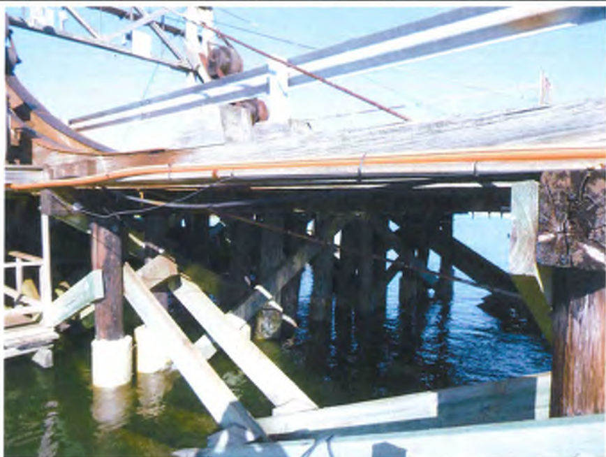
Photo 12 Category: 09 - Utilities/Light Poles Description: South fascia in Span 9, looking northwest. Loose wires and hanging conduit. Moderate rust to conduit.
