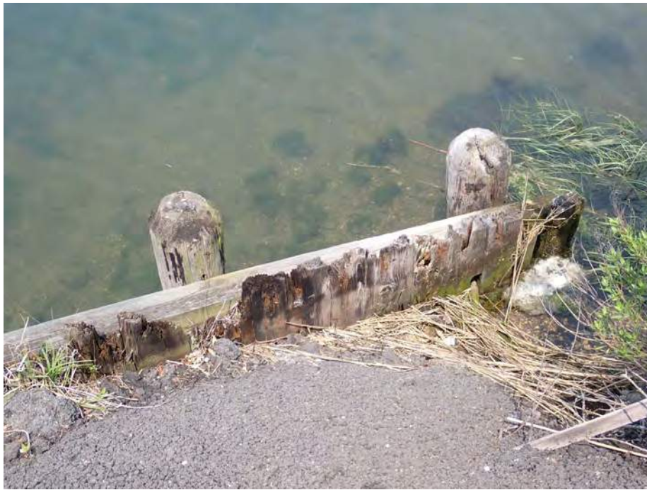
Photo 19 Category: 31 - Wingwalls/Retaining Walls/Headwalls Description: Northwest wingwall, looking west. Advanced decay to top of sheeting.
