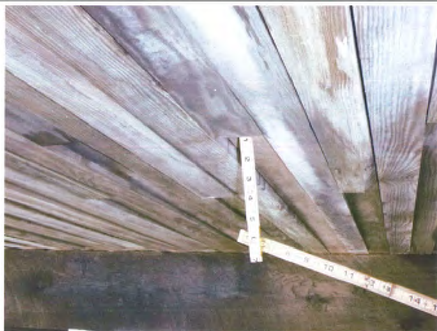
Photo 17 Category: 20 - Superstructure Defects Description: Minor misalignment between deck planks in Span 4, looking west.
