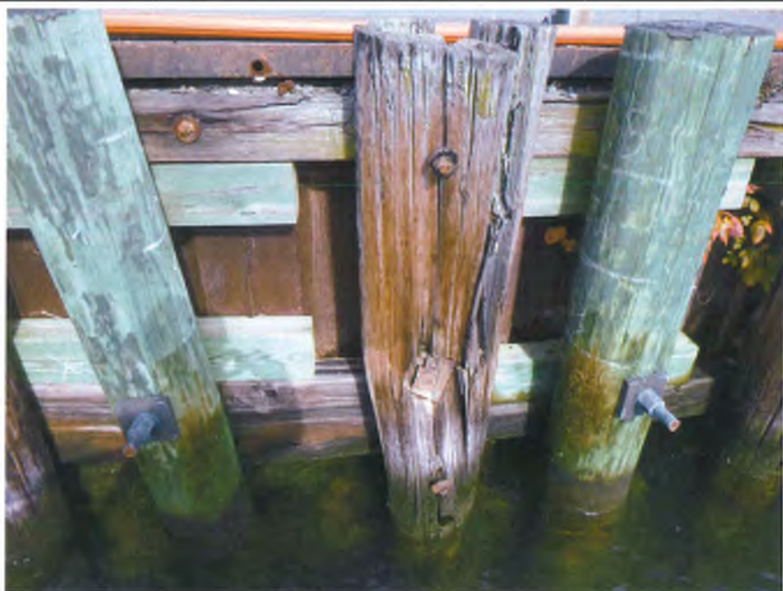
Photo 34 Category: 31 - Wingwalls/Retaining Walls/Headwalls Description: Southeast wingwall, looking north. The 14th pile from the East Abutment is deteriorated.
