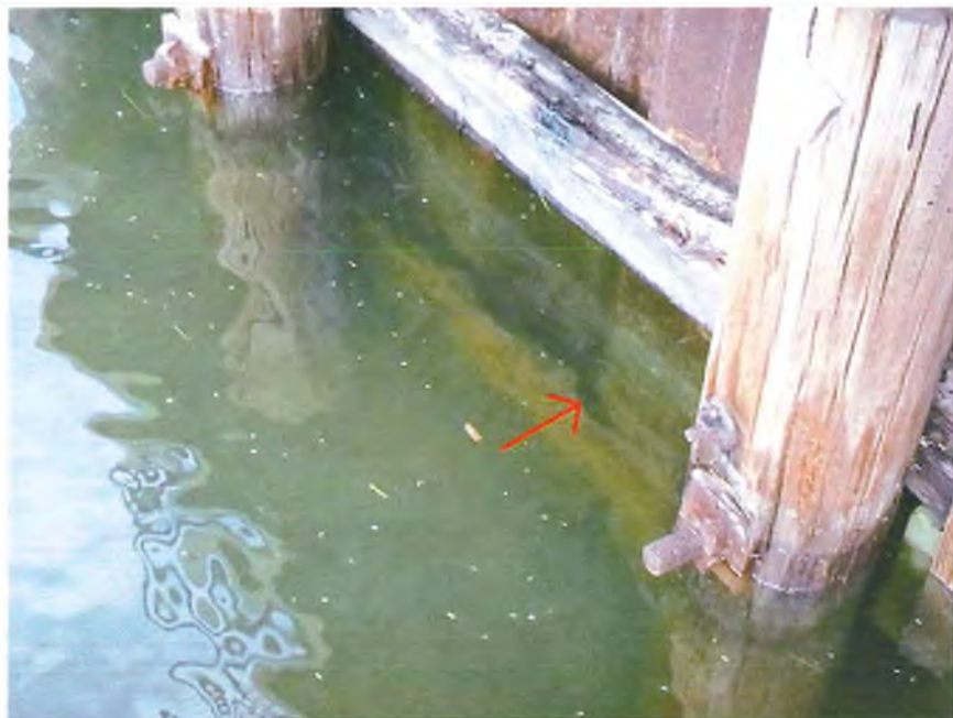
Photo 35 Category: 31 - Wingwalls/Retaining Walls/Headwalls Description: Southwest wingwall between Piles 11 and 12, looking northwest. The water below the water surface is deteriorated.
