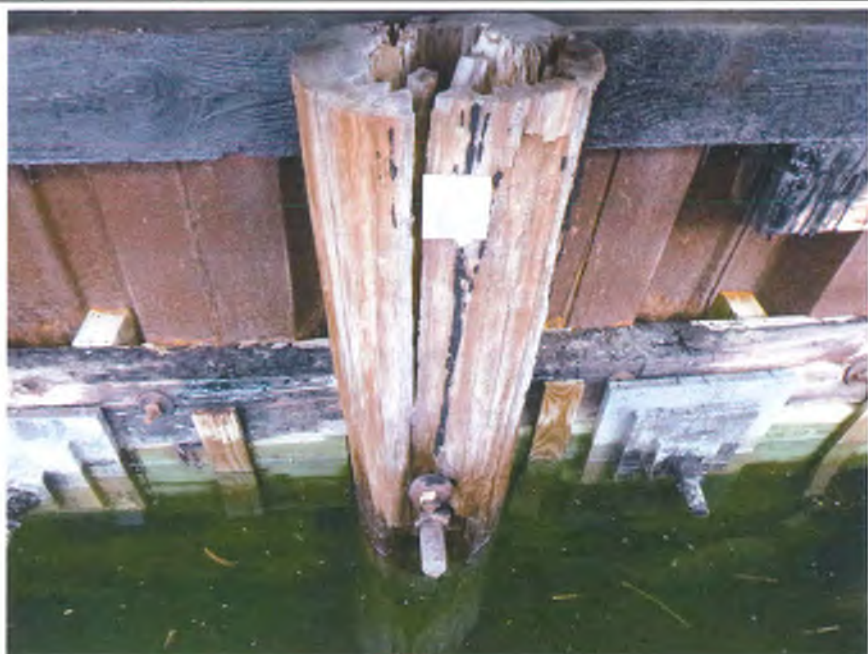
Photo 32 Category: 31 - Wingwalls/Retaining Walls/Headwalls Description: Southwest wingwall, 9th pile from the West Abutment face, looking north. Pile is deteriorated.
