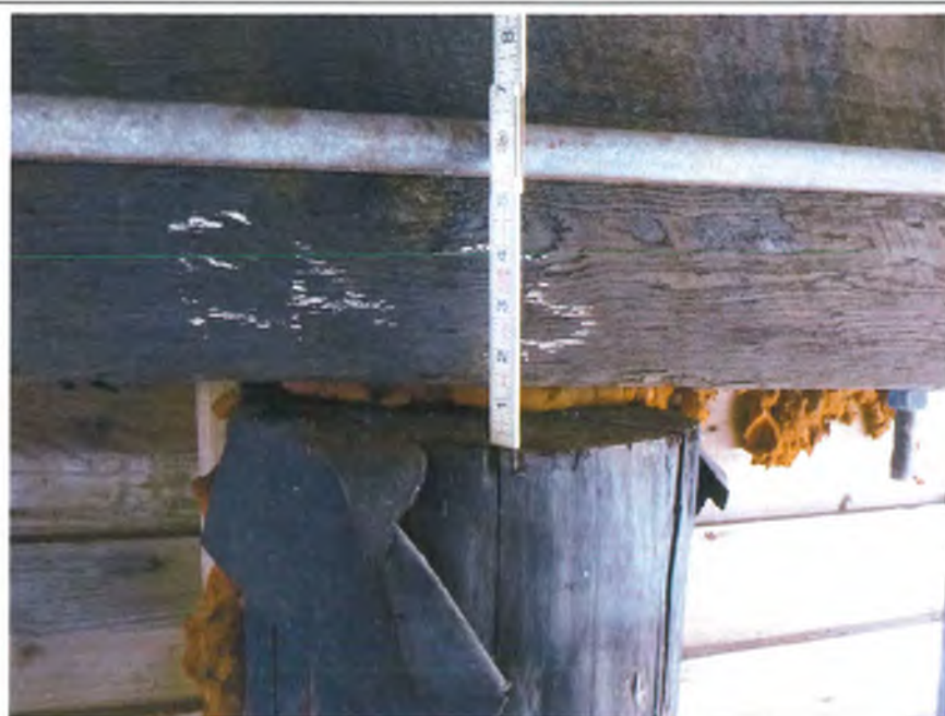
Photo 33 Category: 36 - Piles/Sheeting/Wales Description: Pile 3 at the East Abutment, looking east. 1" gap between the abutment cap and pile.
