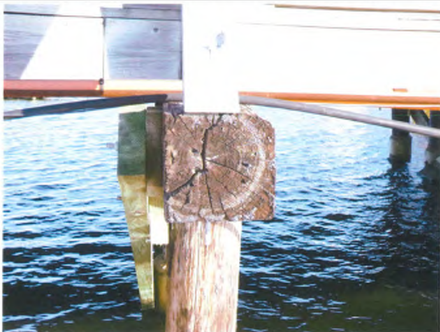
Photo 38 Category: 35 - Pile Bent/Cap/Bracing/Foundation Description: Bent 15 pier cap, looking north. South nose has wide checks.
