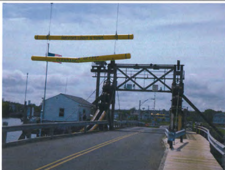
Photo 39 Category: 10 - Signs/Posting Description: East approach spans, looking west. 3 Ton Weight Limit sign and 10 ft Vertical Clearance bar.
