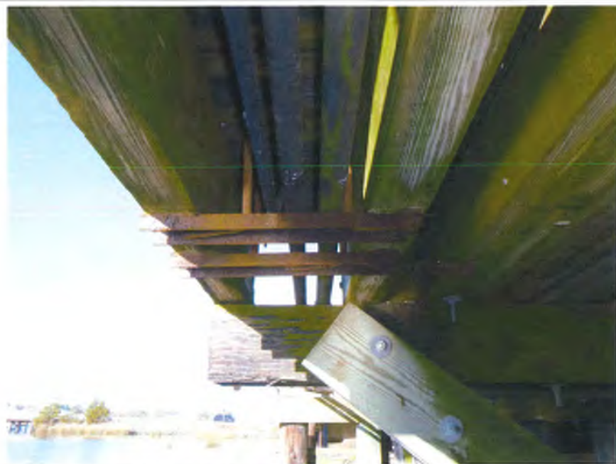
Photo 13 Category: 01 - Deck Defects Description: South fascia lamppost supports, looking west. Supports are severely corroded.
