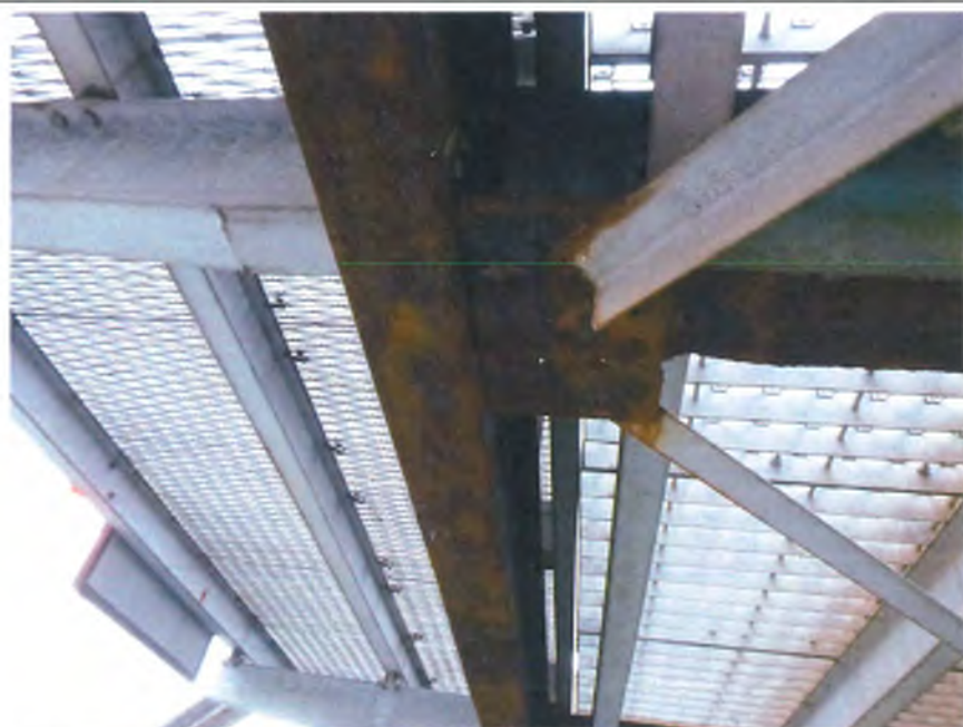
Photo 21 Category: 20 - Superstructure Defects Description: North girder, Span 6, looking east. Typical section loss (1/8") at bottom flange.
