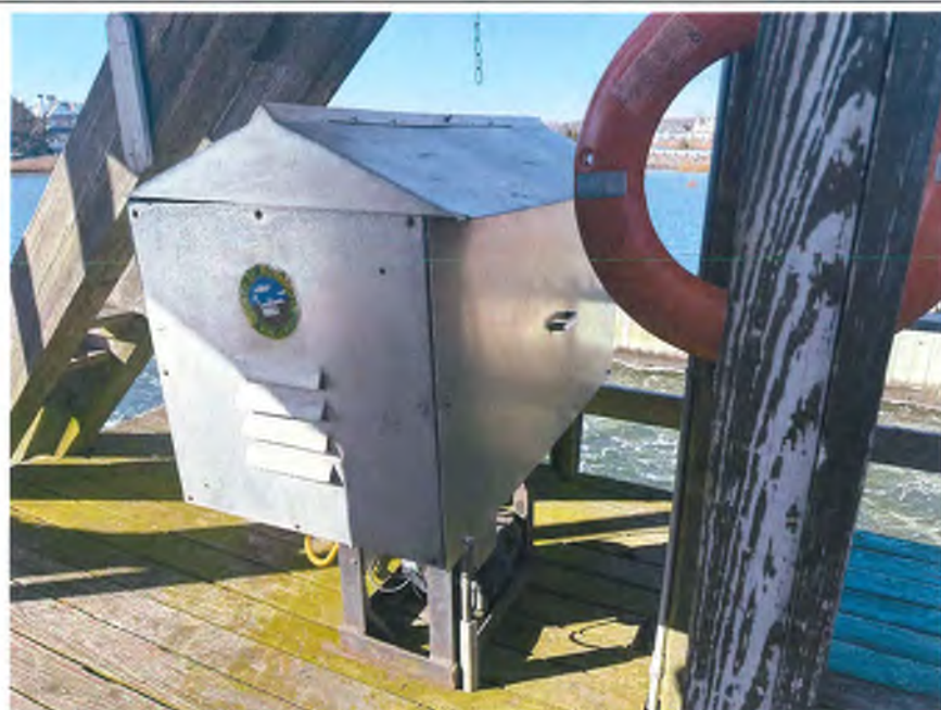
Photo 9 Category: 59 - Other, 60 - Priority Repair Description: Genset on the operator's platform, looking east. Genset is inoperable.
