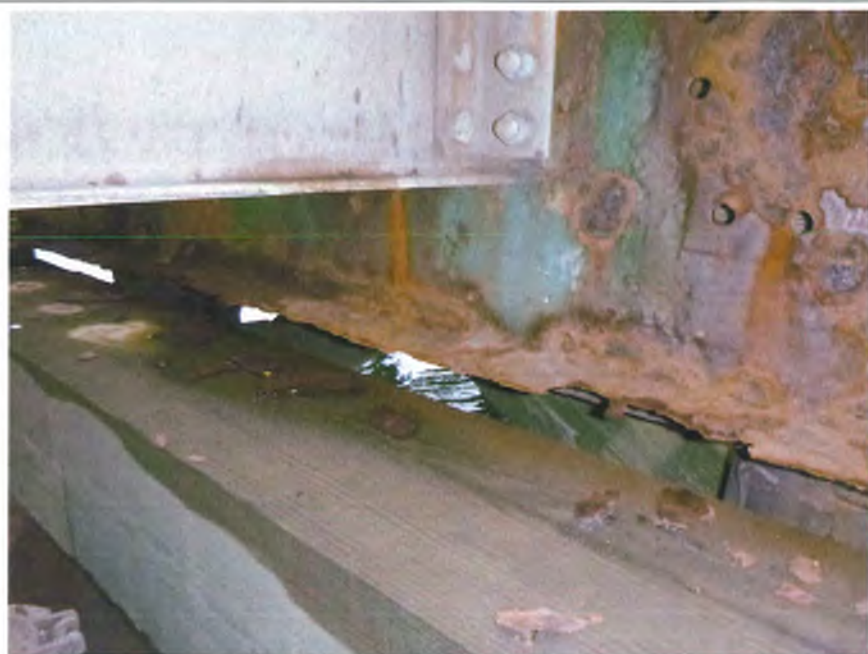
Photo 23 Category: 20 - Superstructure Defects Description: Floorbeam 1 in Span 6, looking southwest. Section loss to bottom flange between Stringers 5 and 7,
