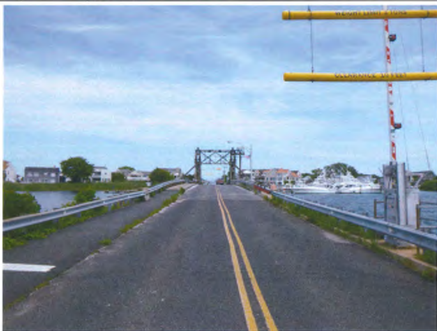
Photo 4 Category: 02 - Approaches, 00 - General View Description: West approach roadway, looking east. Wide cracks in pavement throughout the roadway.
