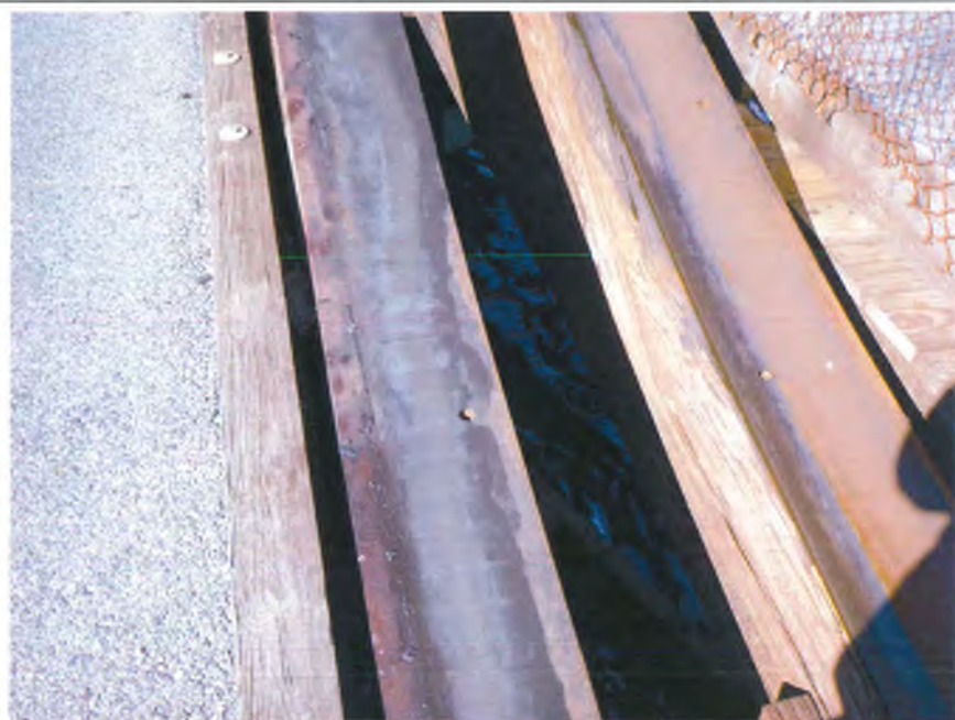
Photo 29 Category: 59 - Other Description: Missing connection bolt in north counterweight track, looking west.
