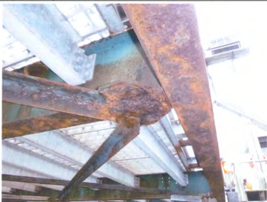
Photo 24 Category: 20 - Superstructure Defects Description: Floorbeam 2 in Span 6, near the South Girder, looking east. Section loss to rivets in connection plate between lateral bracing and floorbeam.
