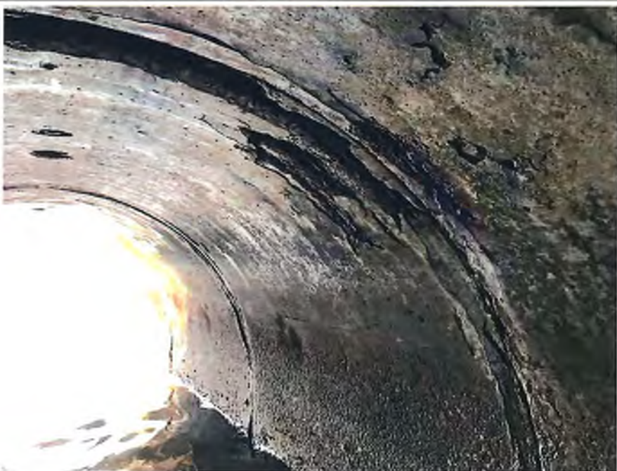
Photo 14 Category: 50 - Culverts/Frames/Arches Description: Joint 5 from west, looking southeast. Note 6 SF spall with exposed corroded rebar that exhibits heavy section loss.
