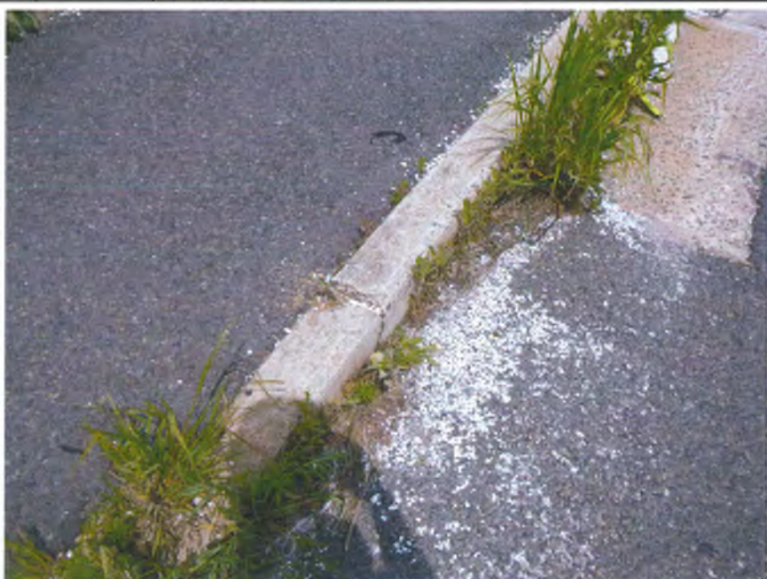
Photo 16 Category: 05 - Sidewalks/Safetywalks/Curbs, 02 - Approaches
