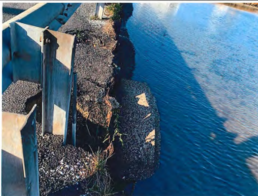
Photo 8 Category: 60 - Priority Repair , 50 - Culverts/Frames/Arches, 51 - Erosion Description: West end of culvert, looking south. Note: Heavy erosion has been noted above west end of pipe. (Refer to Priority Repair Letter 2_2022_16941)
