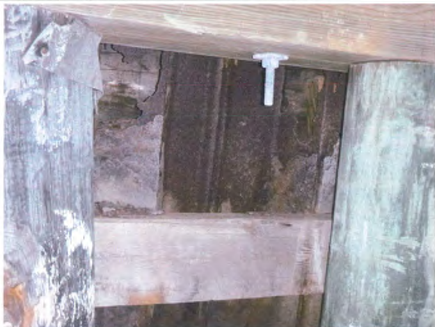
Photo 30 Category: 32 - Substructure Embankment/Slope Protection, 36 - Piles/Sheeting/Wales, 30 - Abutments Description: West Abutment bulkhead sheeting, looking west. Corrosion holes in steel sheeting.
