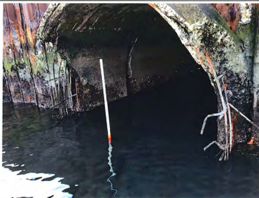
Photo 11 Category: 50 - Culverts/Frames/Arches Description: West end of arch, looking northeast. Note 100% loss of concrete with exposed corroded cage from mud line up to 4' high.
