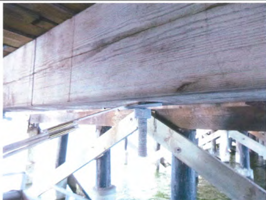
Photo 20 Category: 20 - Superstructure Defects Description: Loose deck hardware between deck and transverse tie in Span 12, looking southwest.
