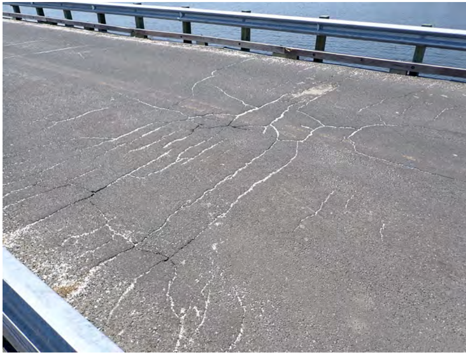
Photo 15 Category: 01 - Deck Defects Description: Top of deck, Span 7S, looking southwest. Moderate wear and medium to wide transverse and longitudinal cracks throughout (typical all spans).
