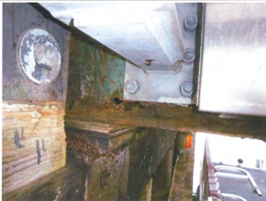
Photo 22 Category: 35 - Pile Bent/Cap/Bracing/Foundation, 20 - Superstructure Defects Description: North girder at the east end, looking south. Hole in web near bottom flange. Masonry plates at Bent 6 are moderately rusted.
