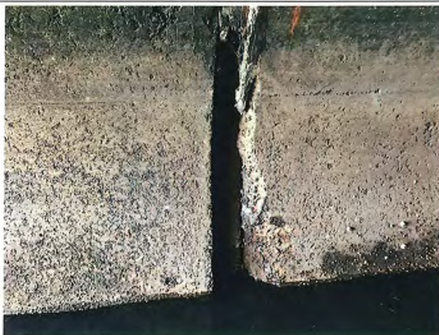
Photo 13 Category: 50 - Culverts/Frames/Arches Description: Segment 4, joint 4 looking north. 4 SF spall with exposed corroded rebar that exhibits heavy section loss
