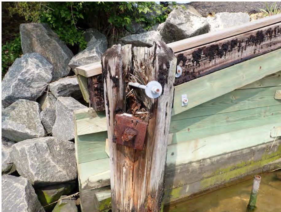
Photo 20 Category: 31 - Wingwalls/Retaining Walls/Headwalls Description: Southeast wingwall, Pile P4 from bridge, looking southwest. Advanced decay and heart rot (42" dp.) at the top and corrosion to tie rod plate.
