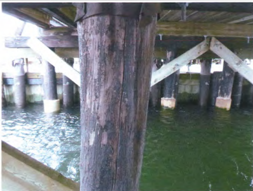
Photo 36 Category: 35 - Pile Bent/Cap/Bracing/Foundation Description: Bent 4, Pile 5, in Span 4, looking east. Surface check in pile.
