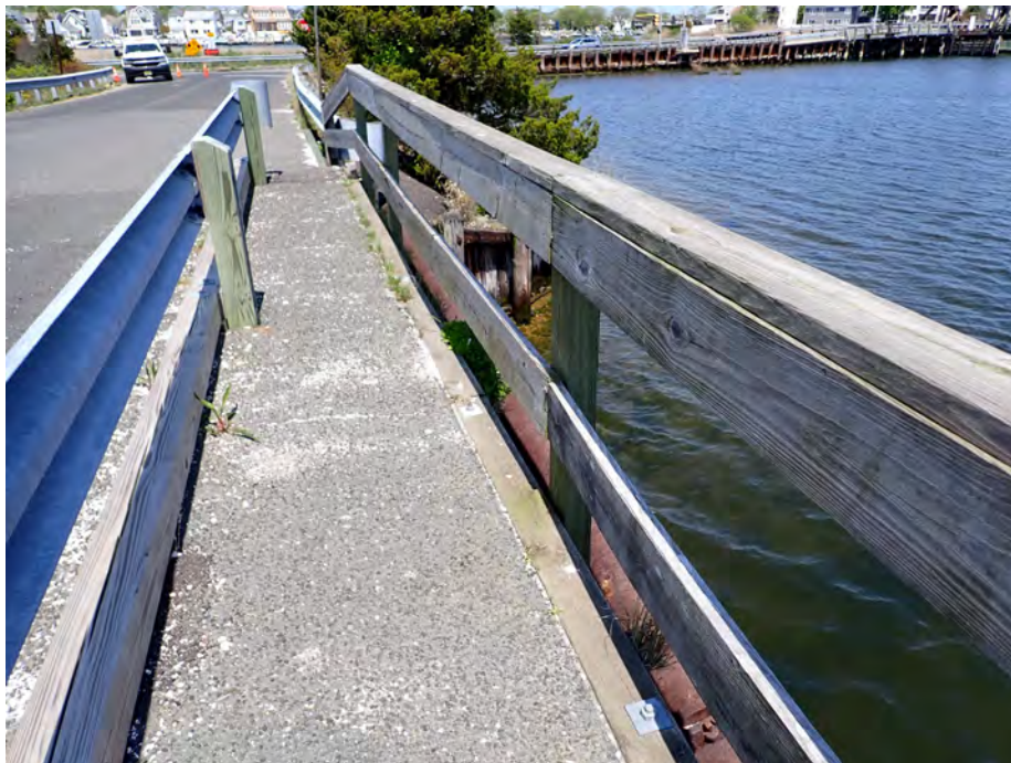
Photo 16 Category: 06 - Parapets/Balustrades/Median/Railings Description: Pedestrian railing, east side, looking north. Posts move due to decay at stringer connection. (Typical)
