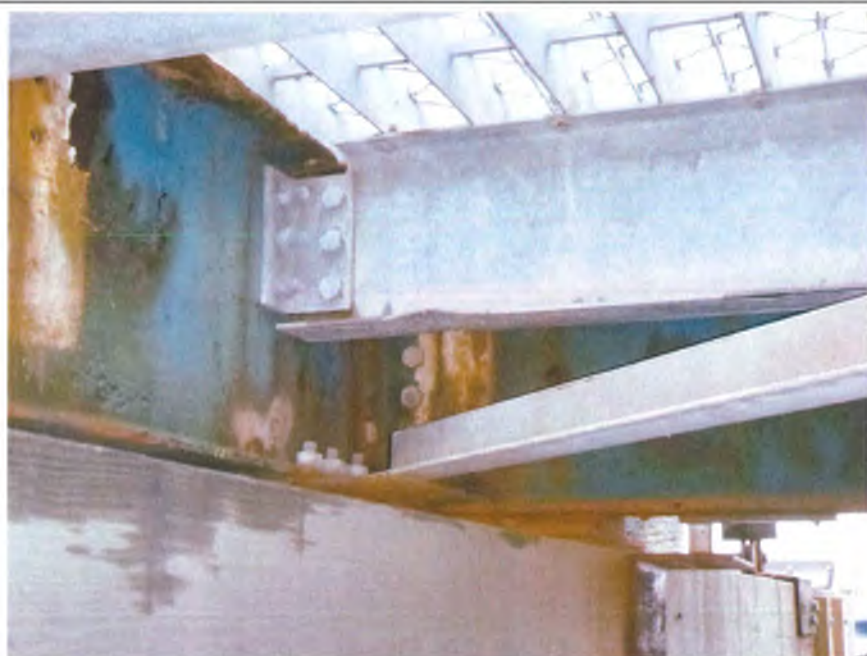
Photo 27 Category: 20 - Superstructure Defects
