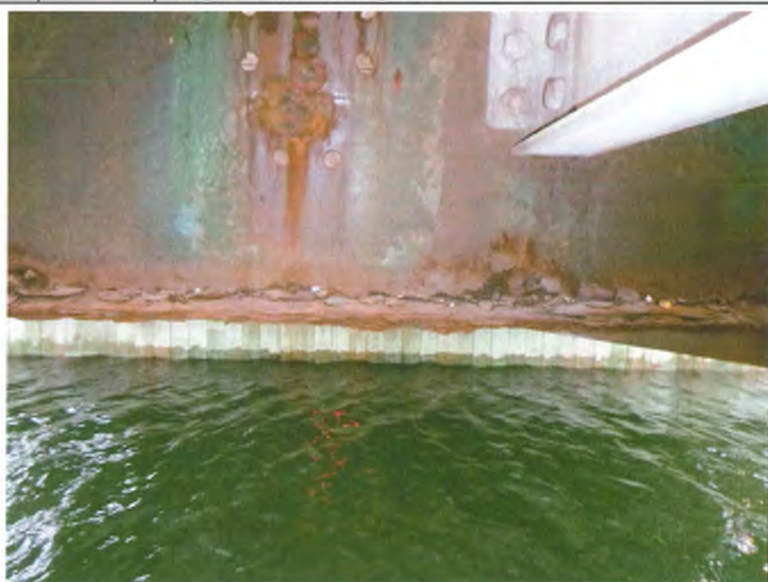
Photo 26 Category: 20 - Superstructure Defects Description: Section loss in bottom flange of Floorbeam 2, in midspan of Span 6, looking east.
