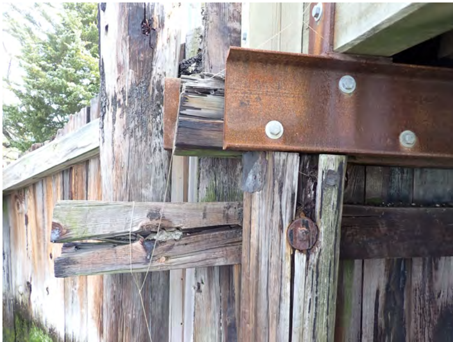
Photo 18 Category: 30 - Abutments Description: North abutment, west end of cap, looking north. Wide split and advanced decay with up to 30% section loss with bolted steel channel. Note wide split to the wale.
