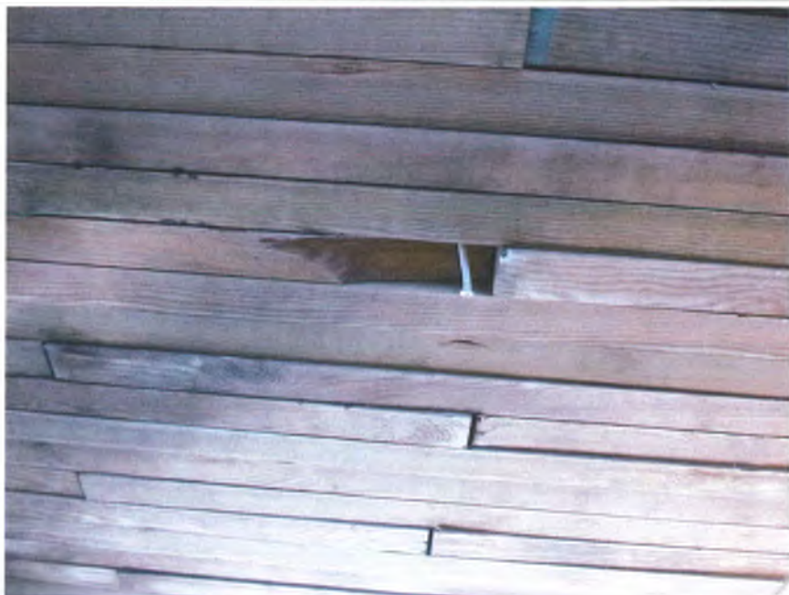
Photo 18 Category: 20 - Superstructure Defects Description: Damaged deck plank and exposed nail in Span 12, looking south.
