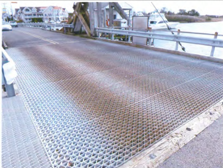
Photo 10 Category: 01 - Deck Defects Description: Top of deck in movable span, looking southeast. Deteriorated timber along the Bent 5 joint.
