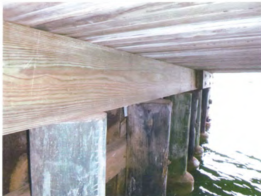
Photo 31 Category: 35 - Pile Bent/Cap/Bracing/Foundation, 30 - Abutments Description: West Abutment, looking northeast. Timber piles are offset up to 5" from pile cap.
