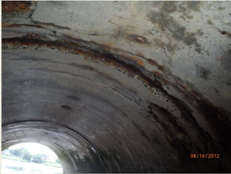
Extensive Cracking in Pipe Walls with Rusting and Exposed Reinforcement
