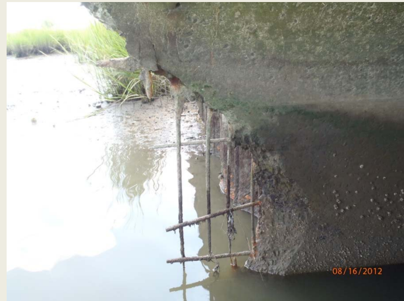
Spalled Pipe Ends with Exposed Reinforcement
