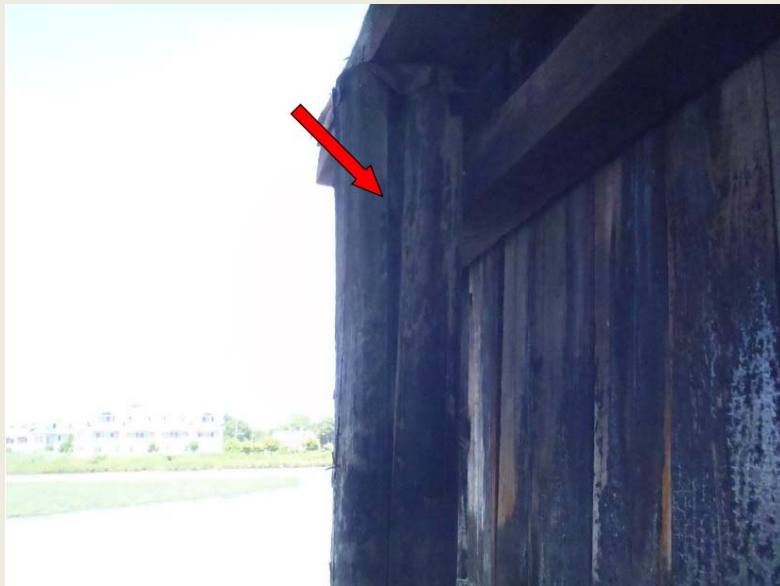
Wide Split in Pile
