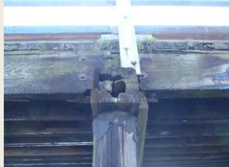
Heart Rot in Pile Bent Cap
