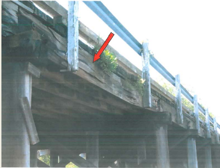
Splits and Sagging in Timber Stringers and Pile Bent Cap
