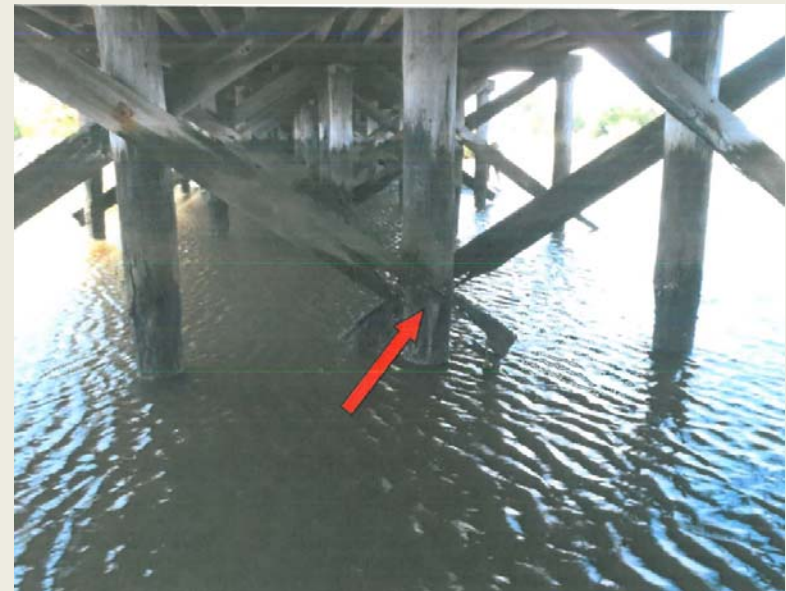
Severely Decayed Pile Bracing and Reduced Pile Cross Sections at Waterline
